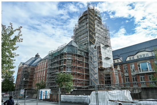
Photo 9: Restoration site at TU Dresden (1): Semi-enclosed construction fencing with dust screens installed only on parts of the scaffolding.
