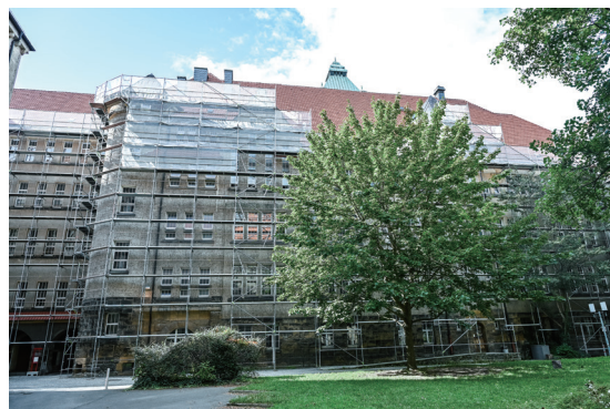
Photo 10: Restoration site at TU Dresden (2): No construction fencing was installed at the site, and dust screens were installed only on parts of the scaffolding.
